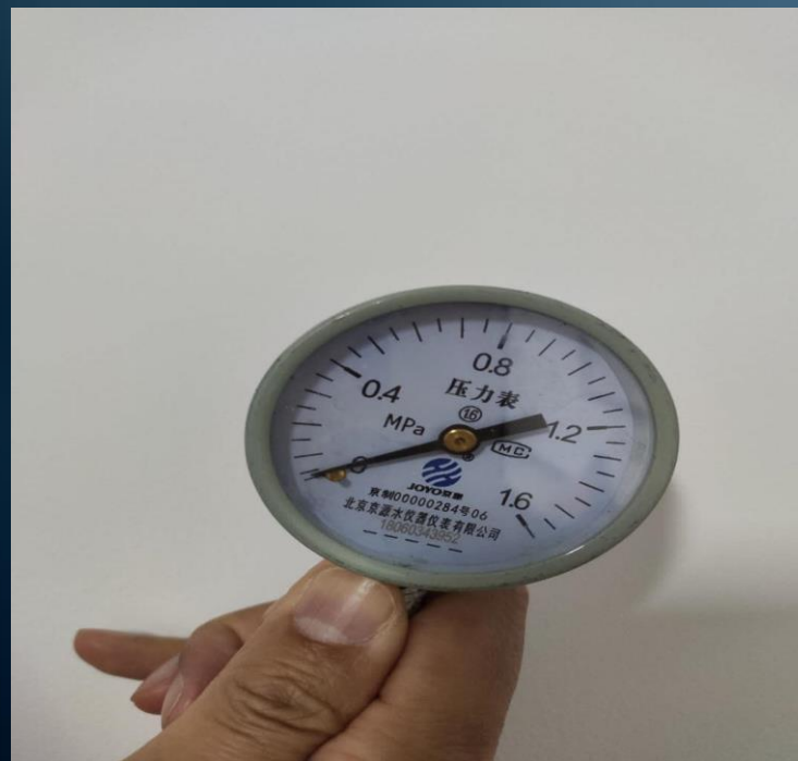
喷淋水管压力为零
